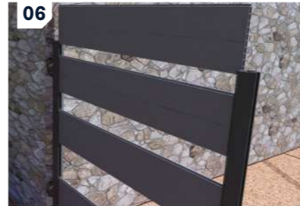
06: Slot in the first fencing board, ensuring it is level before adding the other boards. Each board should sit firmly on the last, similar to tongue and groove.
