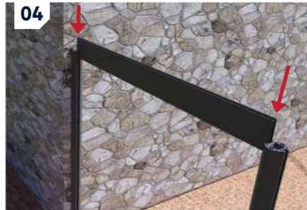
04: Insert the gravel board at the top of both posts and slide it down to the ground.
